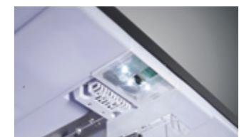
Interior LED light
